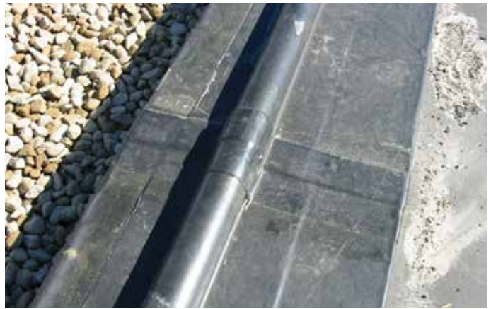
Field fabricated expansion joint
